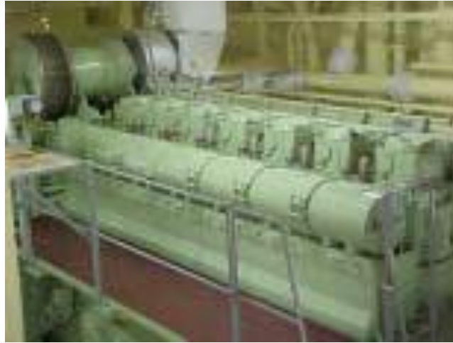
Figure 1-4: One of three (3) MAN B&W 7L32/40, 4-cycle, 720 RPM 3,270 kW Auxiliary Engines connected to the scrubber
