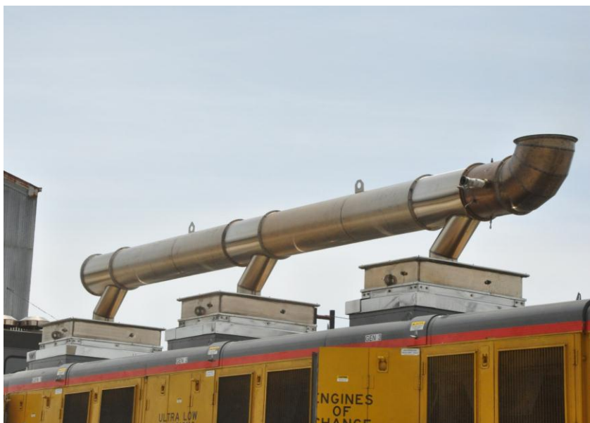
Figure 9: UPY-2755 equipped with 3 L-CCRT's. Exhaust Flow is combined for Part92b Testing
