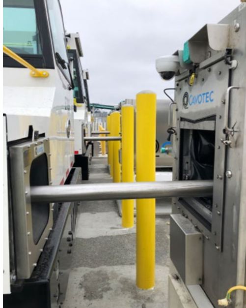
Figure 3: BYD Battery-Electric Yard Tractors Engaged with Cavotec Smart Plug-In System
