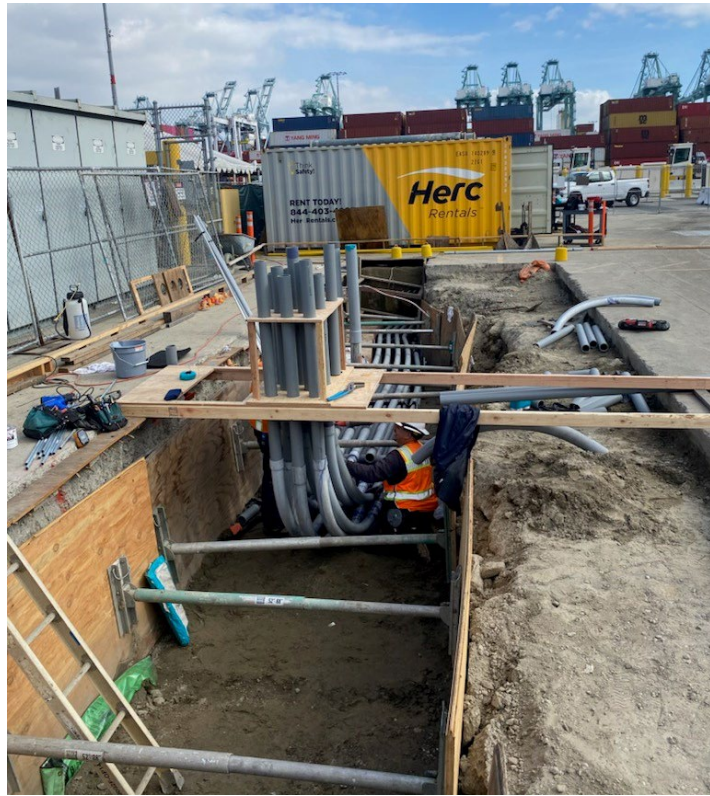
Figure 2: Infrastructure Construction at the Main Equipment Corral: Substation Power Distribution 3-Inch Conduit Placement
